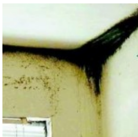
Mold at Bart's Apartments. Photo/South Lake Tahoe
