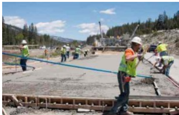
Workers form new concrete on a segment of Interstate 80 near Emigrant Gap and Cisco Grove. Photo/Caltrans
