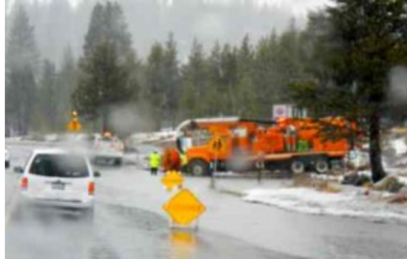
Caltrans works on the flooding issue in Meyers on Feb. 9. Photos/Kathryn Reed
