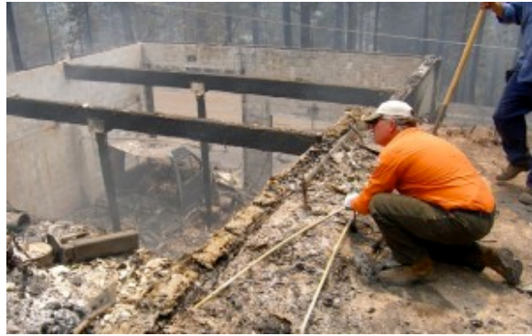
South Tahoe PUD crews repair water supply lines in the Angora burn area. Photo/STPUD
