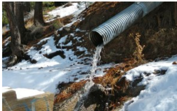
Water flows from the pipe below the old Alta Mira building in South Lake Tahoe. Photo/LTN file
