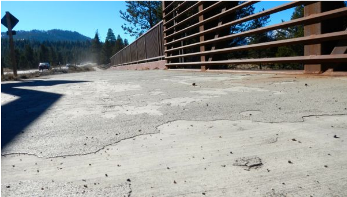
Sawmill bike bridge is in need of a new overcoat. Photo/Kathryn Reed
