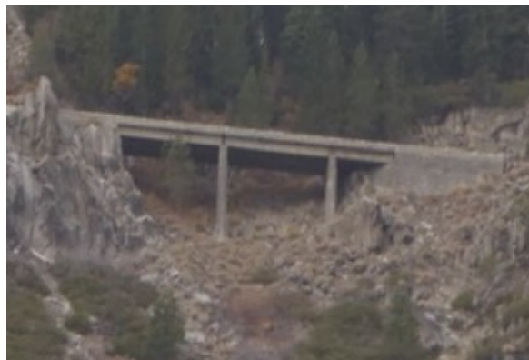
The Highway 50 bridge at Echo Summit is crumbling. Photos/Caltrans
