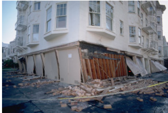
The San Francisco Marin District after the 1989 Loma Prieta earthquake. Photo/J.K. Nakata, U.S. Geological Survey
