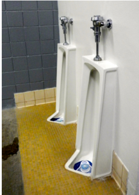
The men's bathroom reflects the age of the facility. Photo/LTN file
