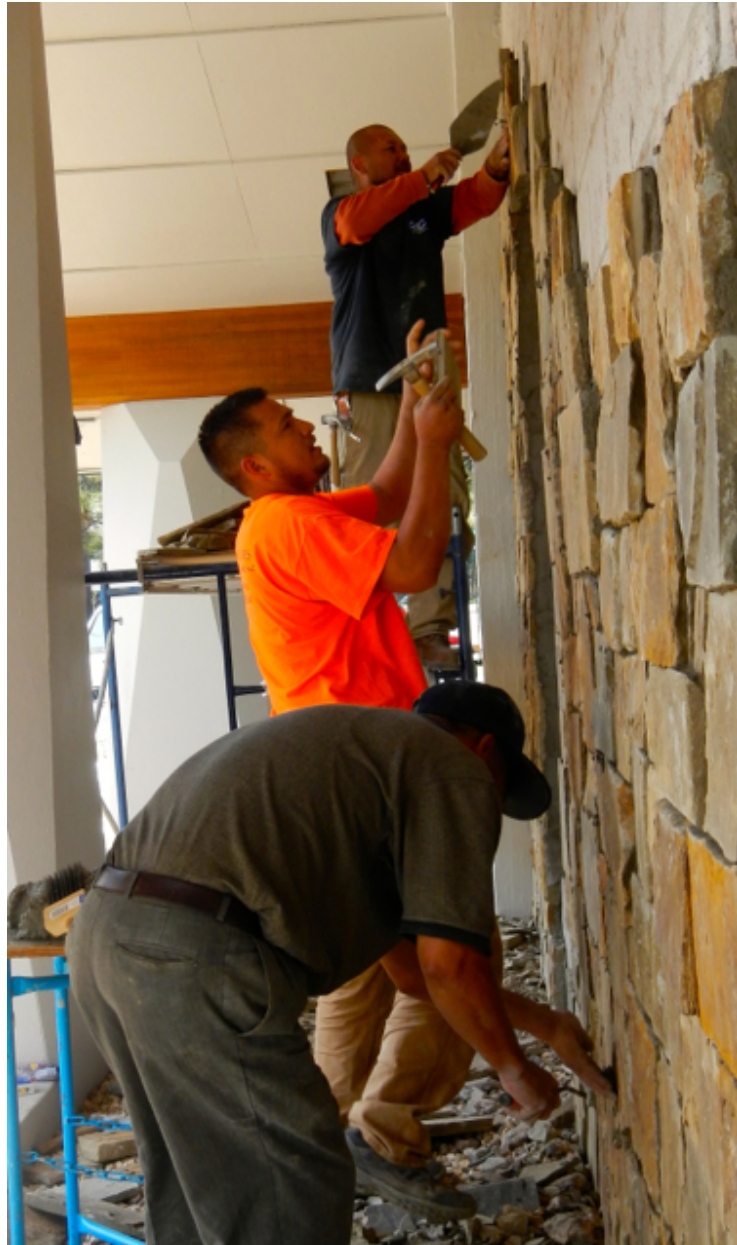
Jose Ribera-Quinonez, Rafael Ayon-Meza and Ceja Gonzalo create a new look for an old building. Photo/LTN
