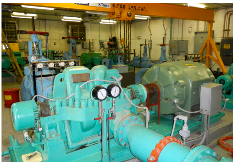
Luther Pass pump station is part of
