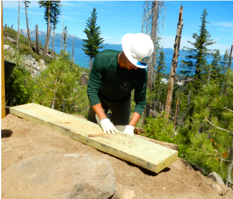
Chris Binder creates a landing area to store the cement. Photo/Kathryn Reed
