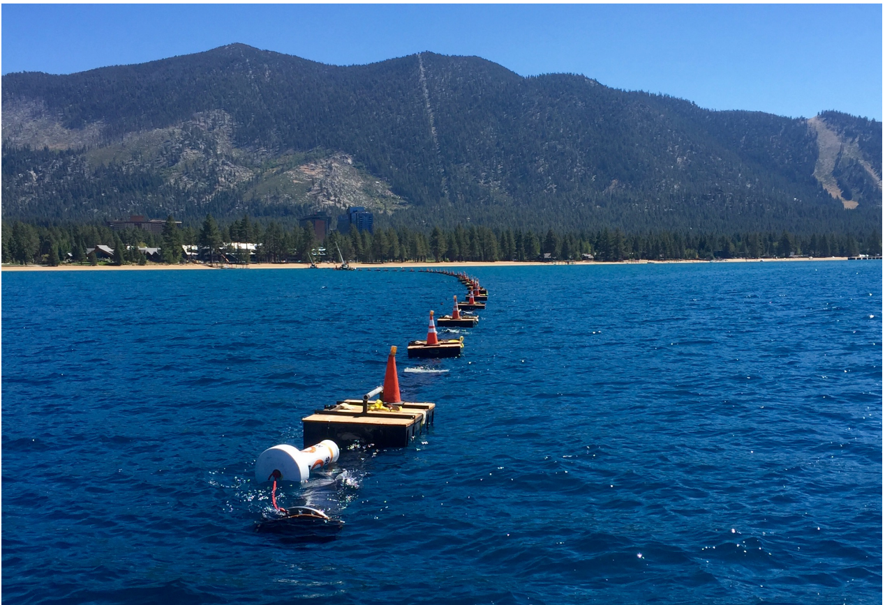
Edgewood Water Company is extending the in-take line 3,000 feet into Lake Tahoe. Photo/LTN
