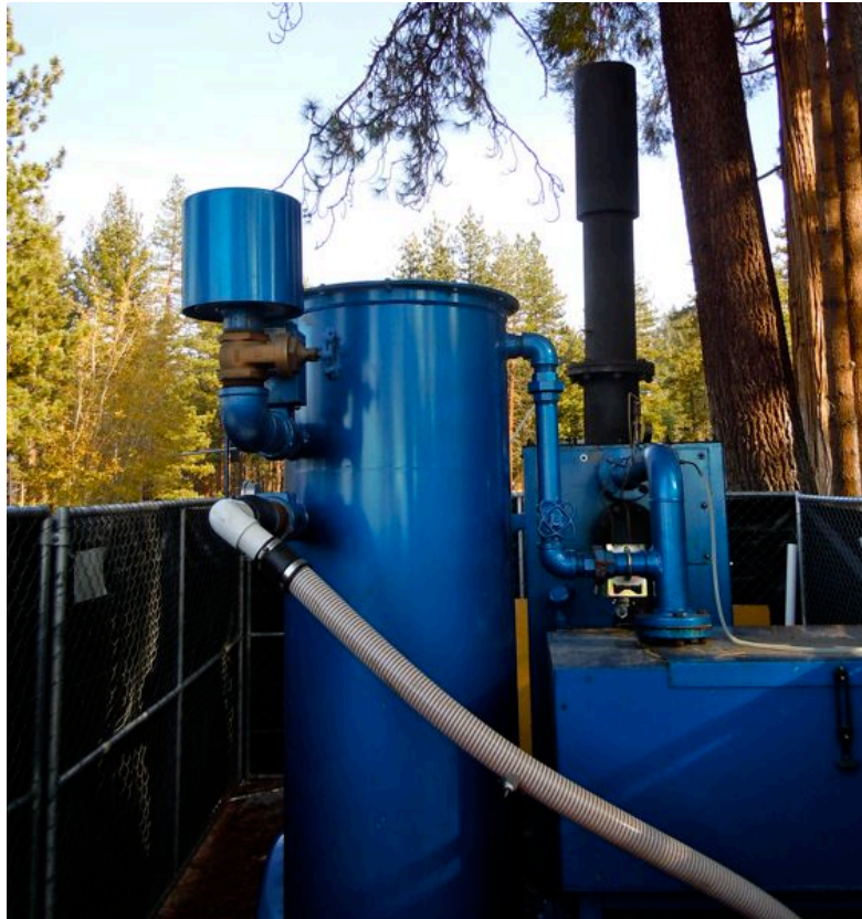
A sparge unit injects air into the soil to get the vapors out. Photo/LTN file
