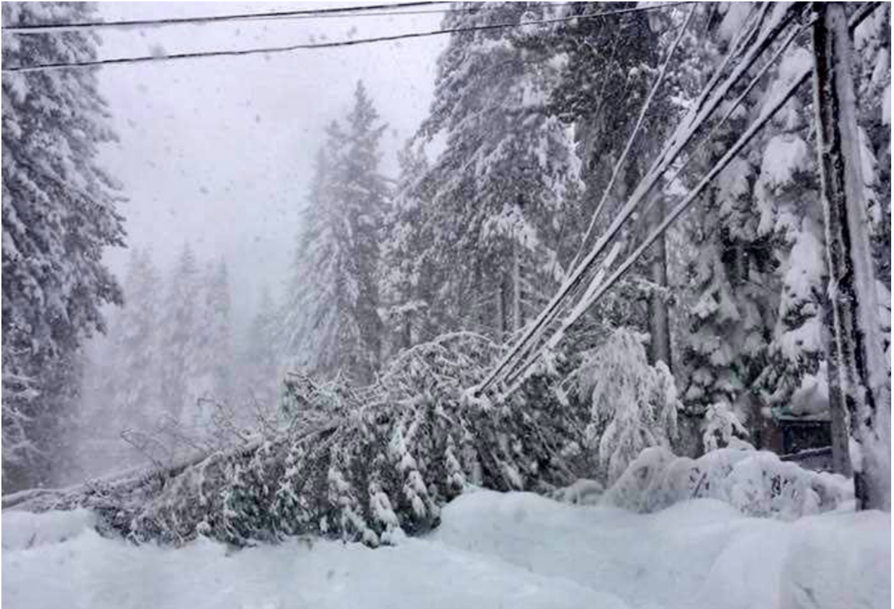
Downed power lines in Incline Village because of toppled trees. Photo/Washoe County
