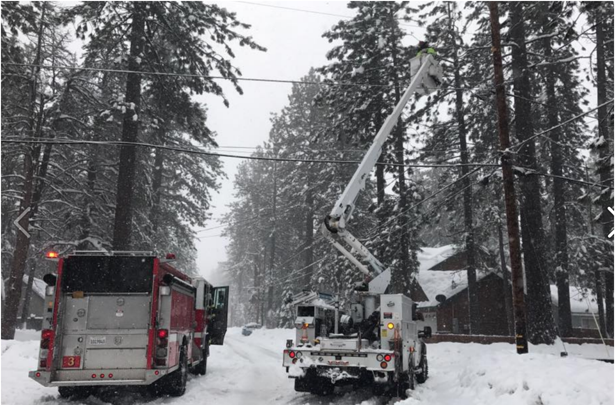
South Tahoe fire and Liberty Utilities crews work on downed power lines. Photo/Provided
