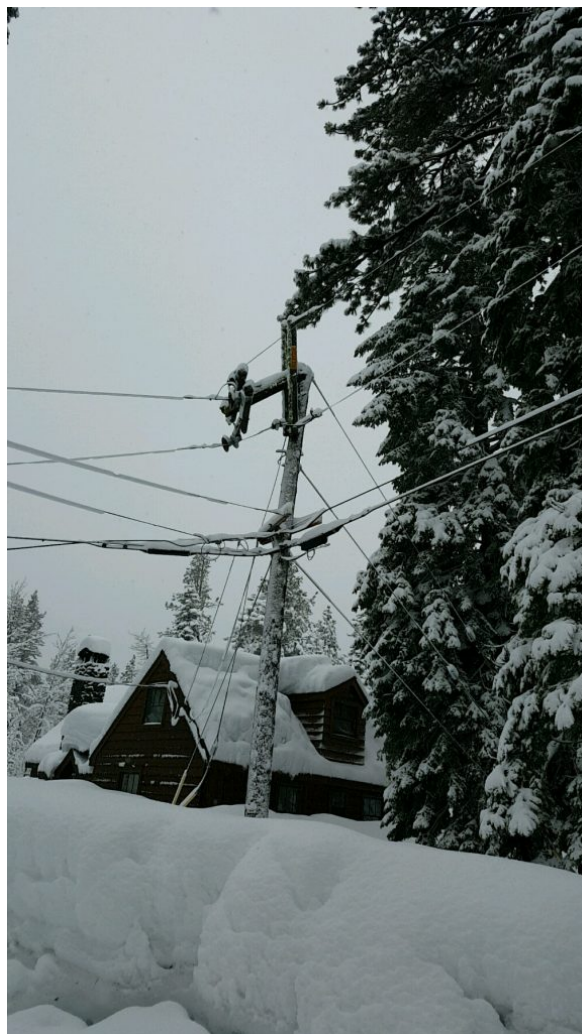
A broken pole in Ward Canyon took out service to part of Alpine Meadows on Feb. 21. Photo/Provided
