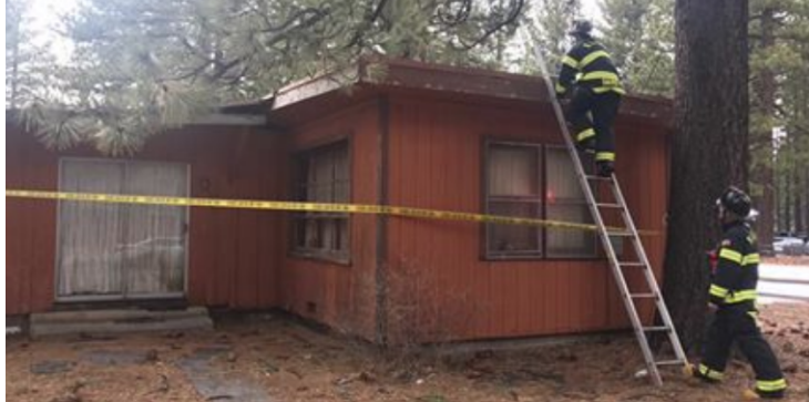
Firefighters on April 11 assess the roof damage. Photo/SLTFD
