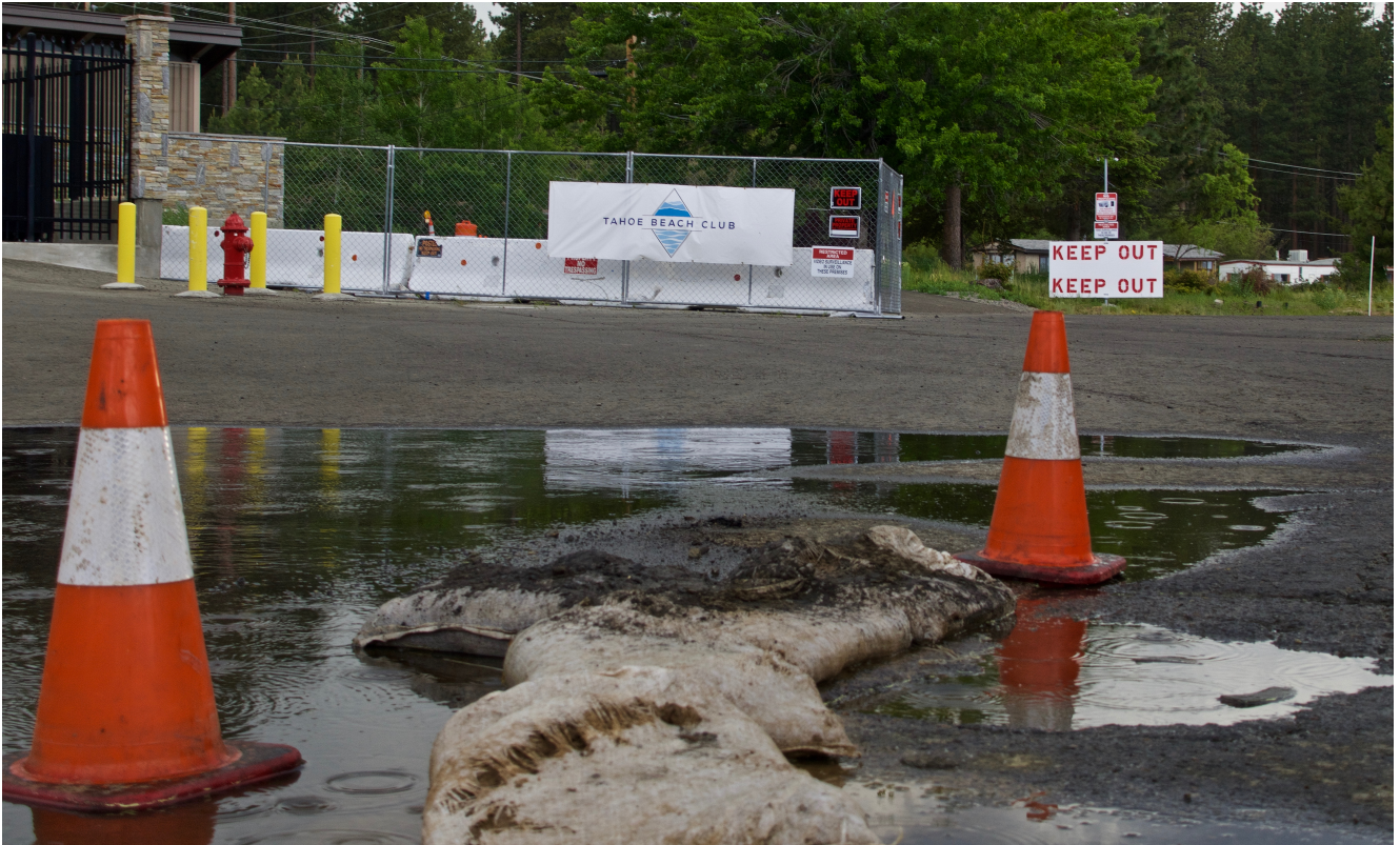
Potholes mar the entrance to the Tahoe Beach Club construction site on Kahle Drive. Photo/Kathryn Reed
