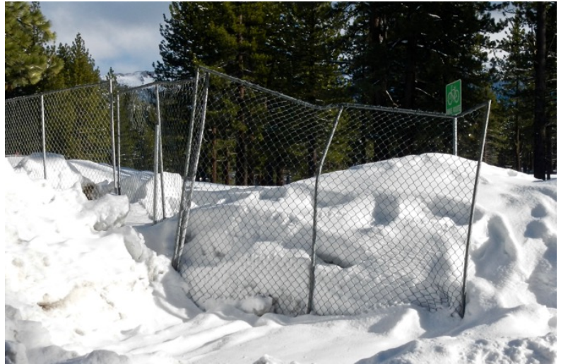
Damaged chain link fences remained for months after SnowGlobe 2016. Photo/LTN
