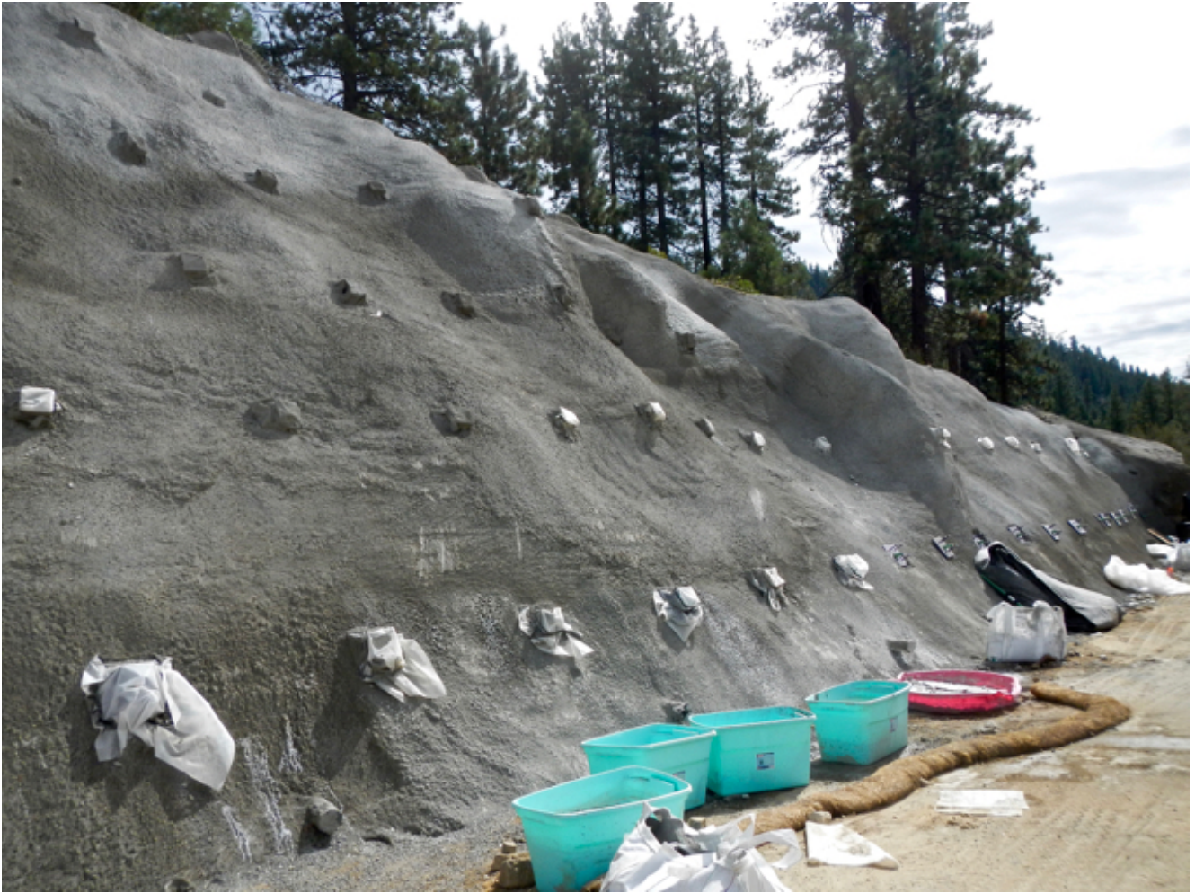
A section of the hillside with the 4-inch concrete spray and limited contouring. Photo/Kathryn Reed
