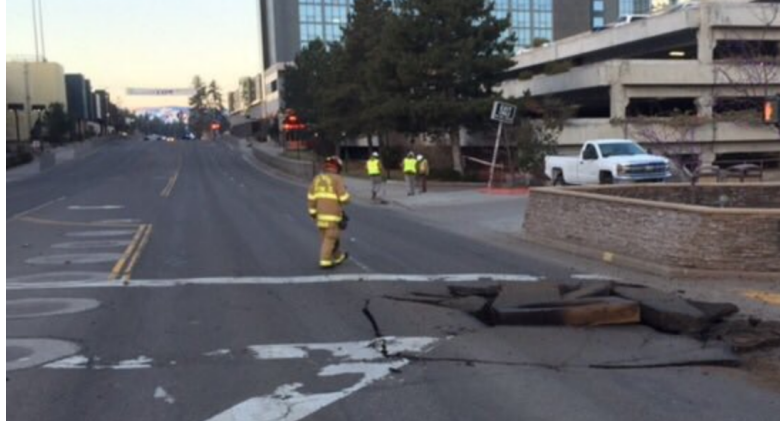
Highway 50 near Hard Rock in Stateline is severely damaged. Photo/DCSO
