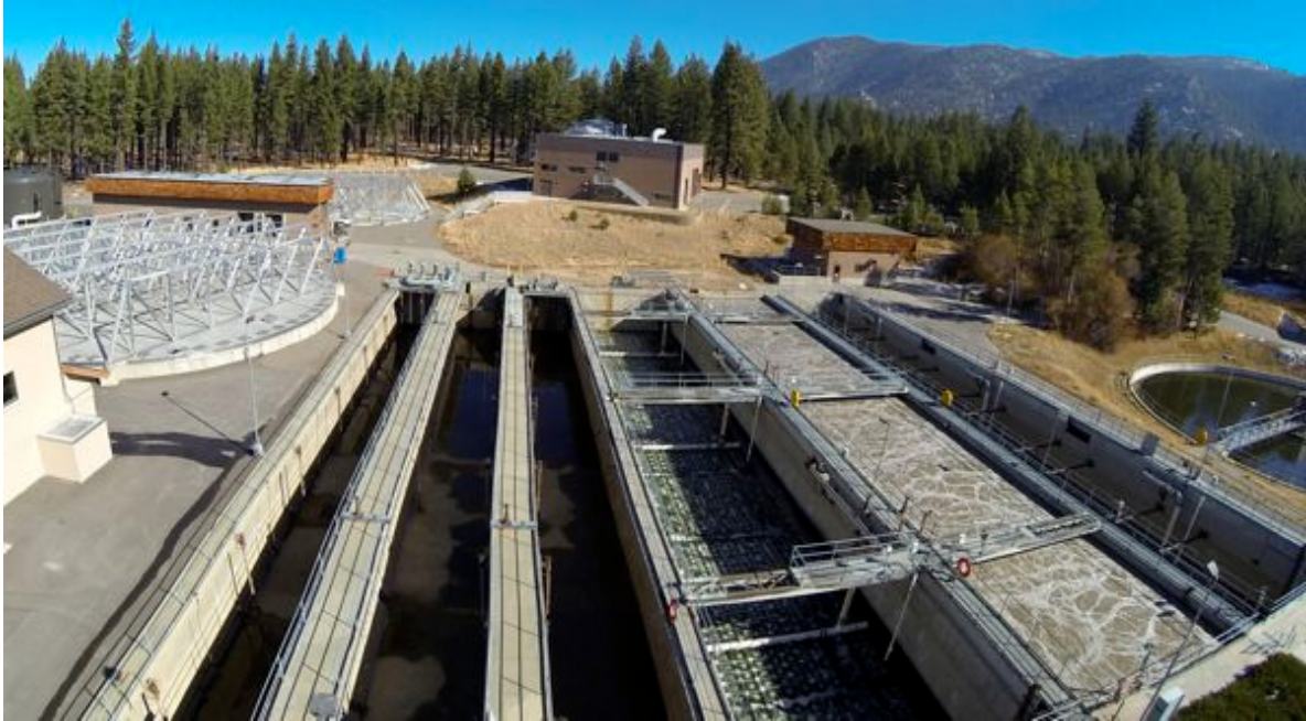
The aeration basin at South Tahoe Public Utility District. Photos/Ross Johnson
