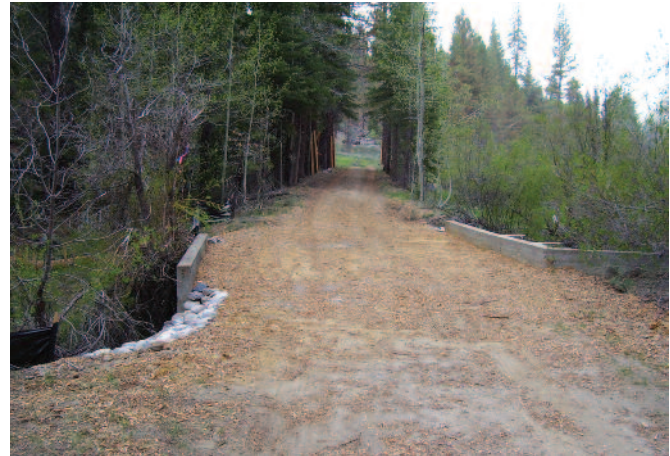
Roads on forest lands are retrofitted with erosion control measures under the EIP.
